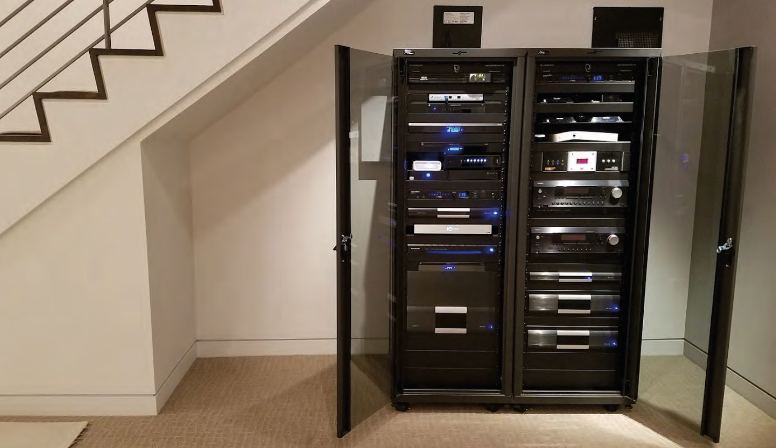
COMPLETED EQUIPMENT RACK
